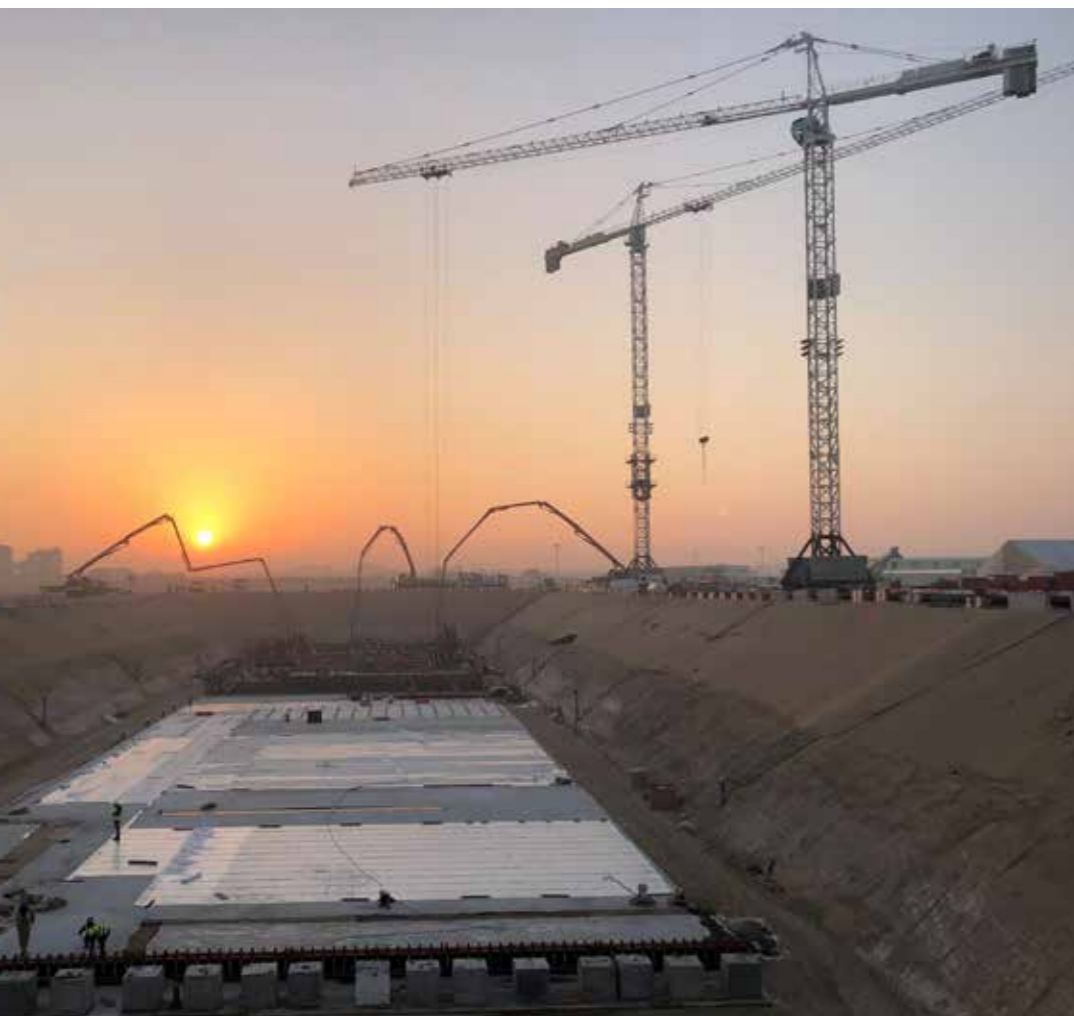
WASTE-TO-ENERGY FACILITY, DUBAI, UAE
